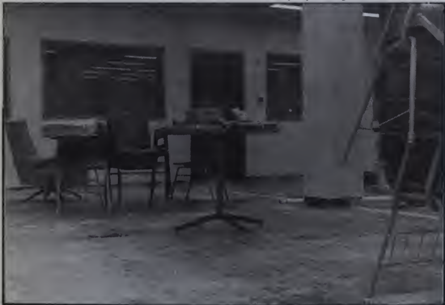
Construction continues in the new sociology department lab center, making room for all the expected new students photo by Katie Lake
